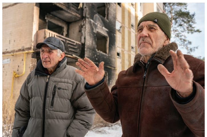
Basil and Nicolai Knutarev stand in front of Basil’s apartment building in Irpin, Ukraine, which was destroyed by Russian artillery in the early days of the invasion. Nicolai’s apartment across the parking lot was also destroyed. (Gregg Brekke)
