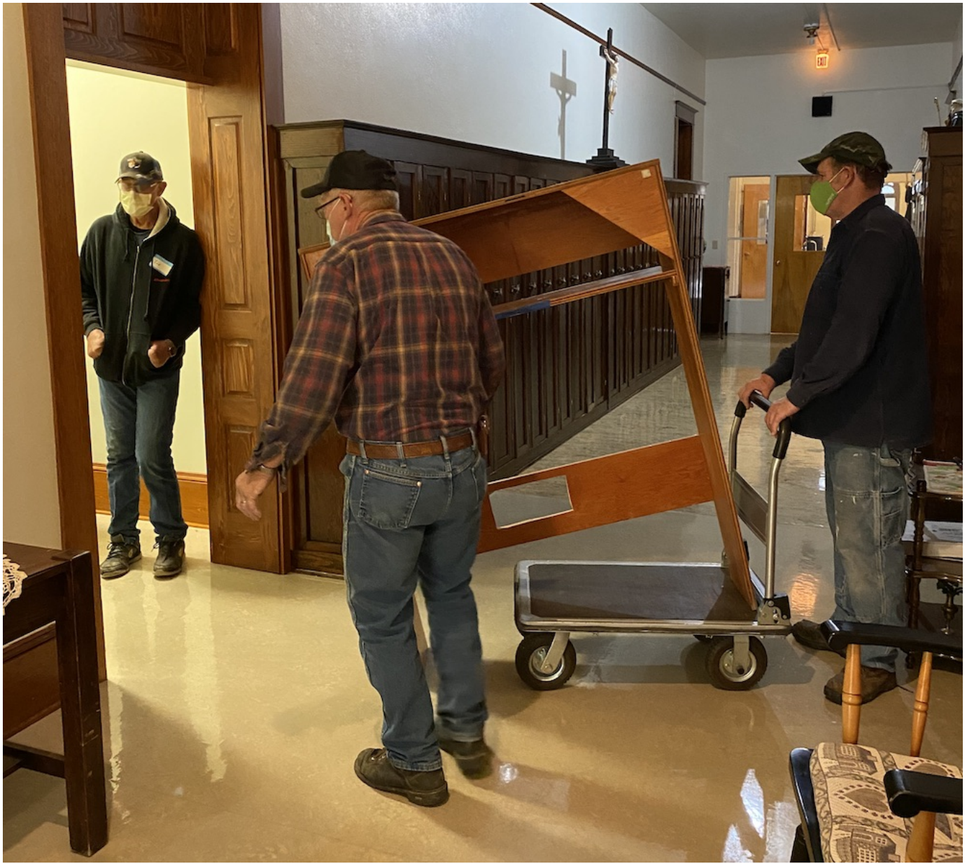
Workers from Arnzen Construction move furniture prior to starting a renovation of the residential Annex at the Monastery of St. Gertrude, Cottonwood, Idaho, in October 2020. (Provided photo)
